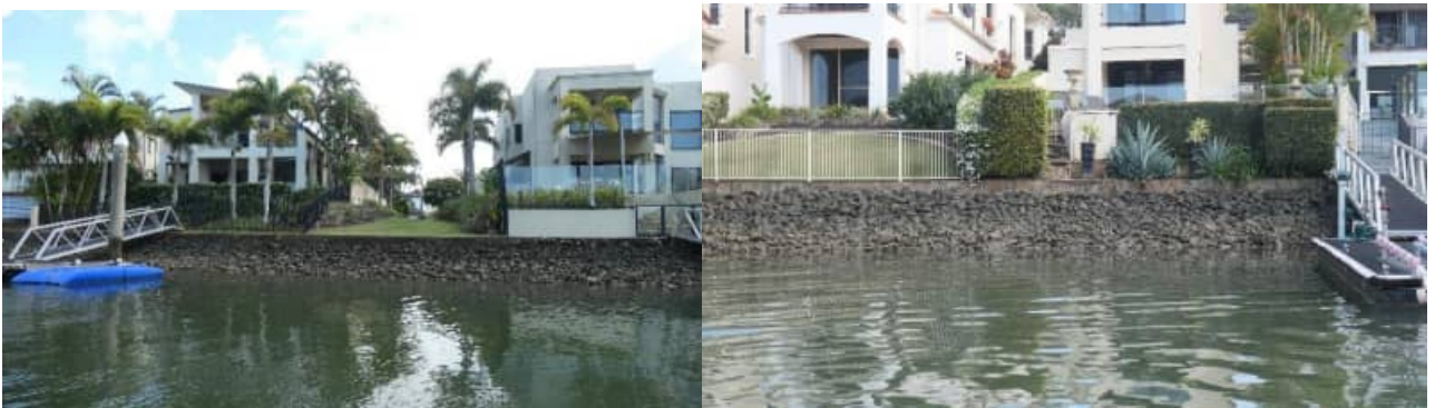
SR-49: example view of revetment wall arrangement / rock armouring to HBR3 – good condition - #3
