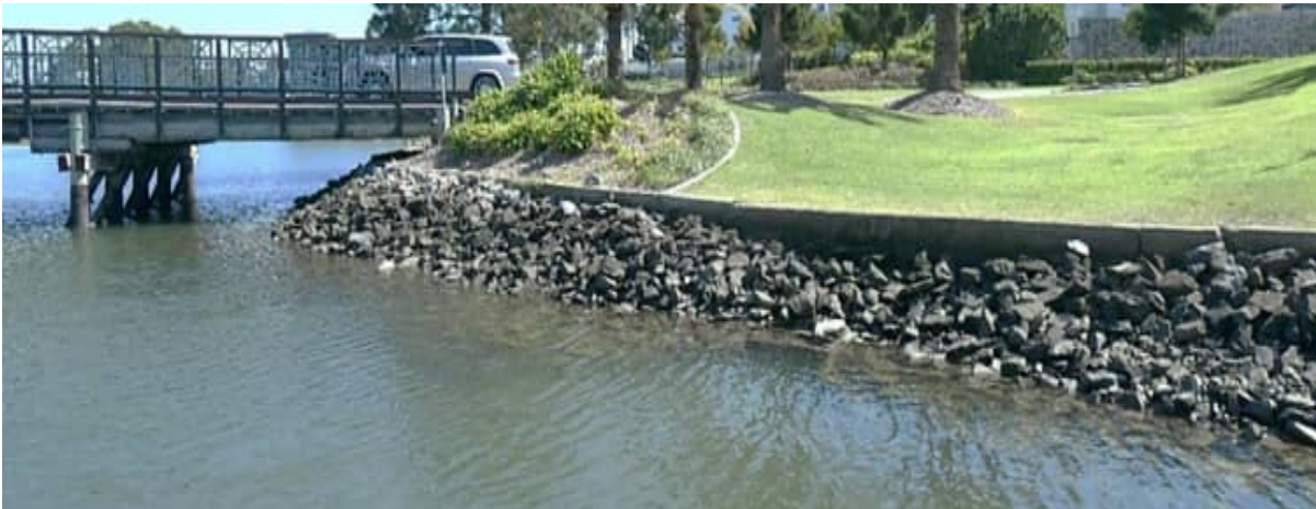
SCB-09: revetment wall arrangement and gabion rock profile adjacent to Western-most RCP outlet
