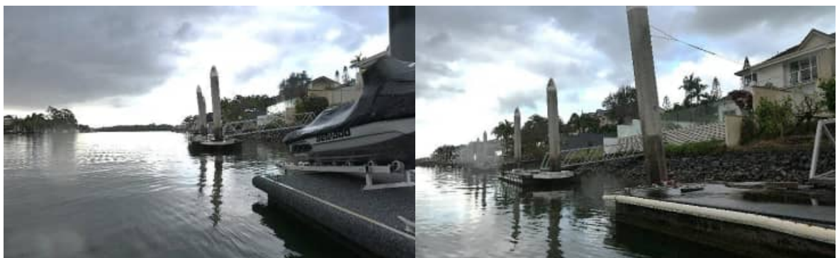
SR-11: 5322 Marine Dve Nth– note pile restraint cables installed to prevent falling
