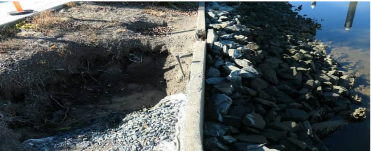
SCC-07: advanced ground subsidence issues about the stormwater RCP - #1
