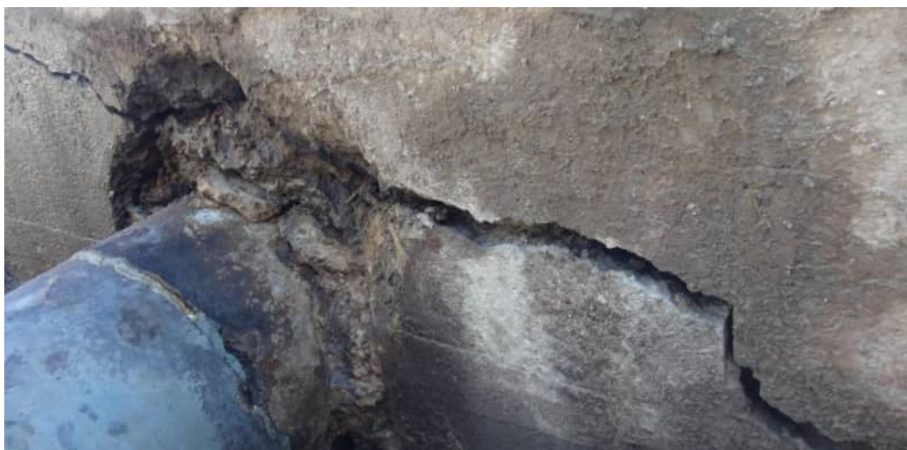
SCB-14: example view of damaged stormwater RCP replacement works (Rabaul Ave Runaway Bay) - #1
