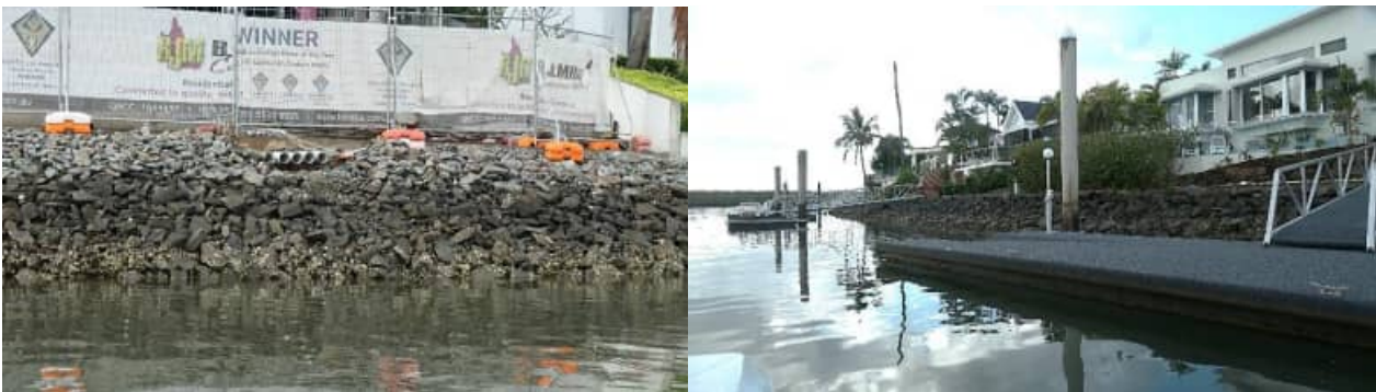
SR-43: example views of generally good condition of revetment wall arrangement / rock armouring to 'Plumeria' - #1
