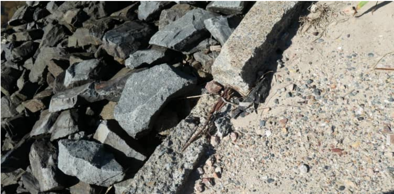
SCE-09: example view of stem deterioration to revetment wall arrangement at easement - #2
