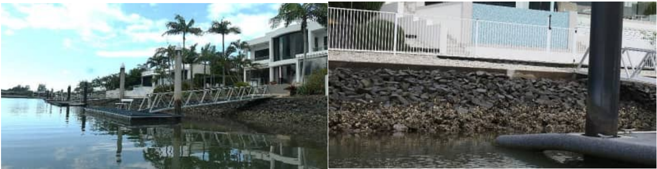
SR-28: example views of Coomera River ('Bauhinia') revetment wall and rock armouring (good) condition – #2
