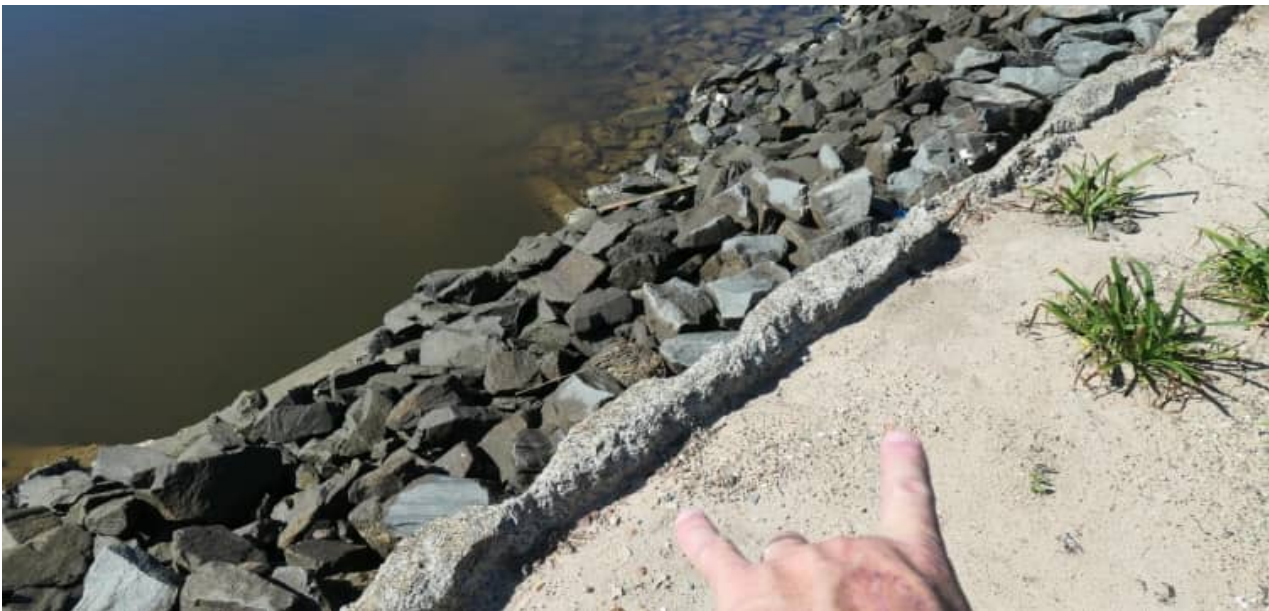
SCE-10: example view of stem deterioration to revetment wall arrangement at easement - #3
