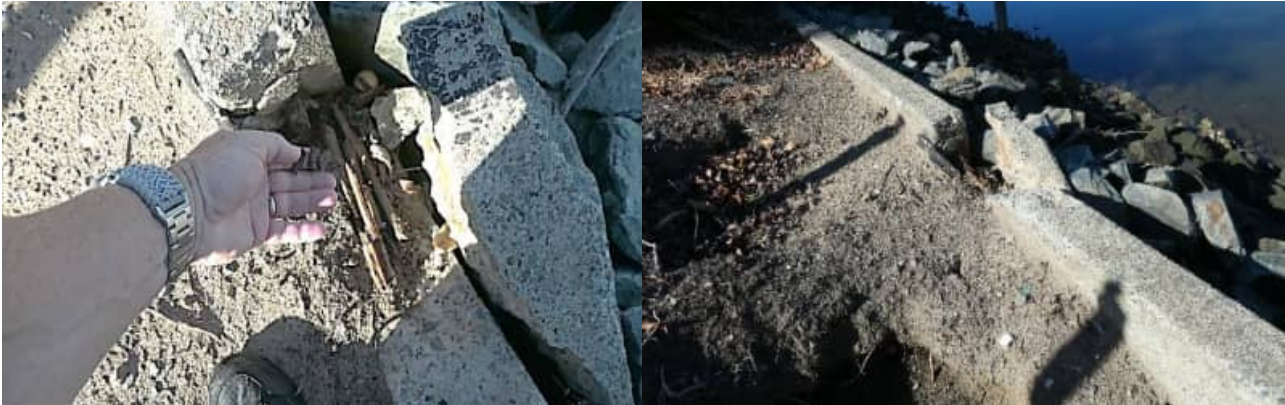
SCC-09: example views of spalling damage to the revetment wall arrangement stem - #1
