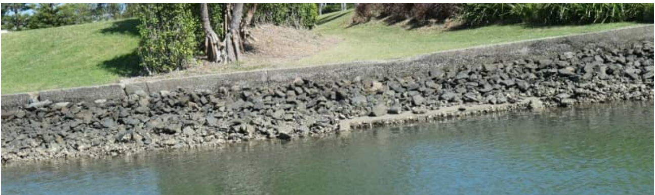
SR-66: example of advancing surface fretting / paste layer deterioration of the revetment wall arrangement stem - #2
