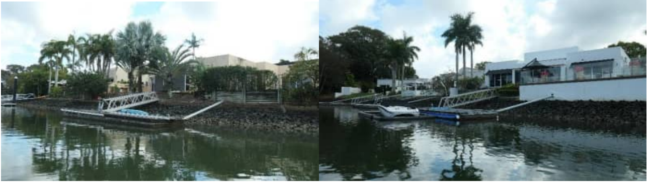
SR-47: example view of revetment wall arrangement / rock armouring to HBR3 – good condition - #1
