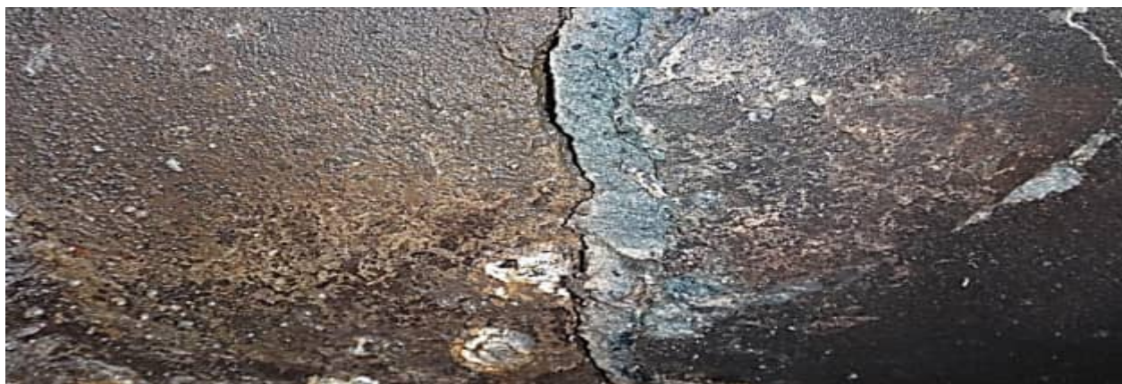
SCC-11: example view of typical subsurface stormwater RCP damage (Rabaul Ave, Runaway Bay) - #1
