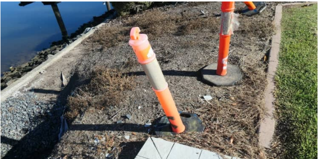
SCC-03: part view of Western batter / canal frontage to the easement between 2026 and 2030 The Circle
