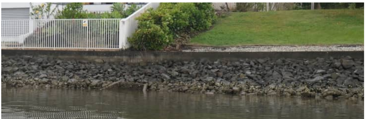
SR-07: shifted / twisted SW outlet headwall to the Easement at (circa) 5252 Marine Dve Nth
