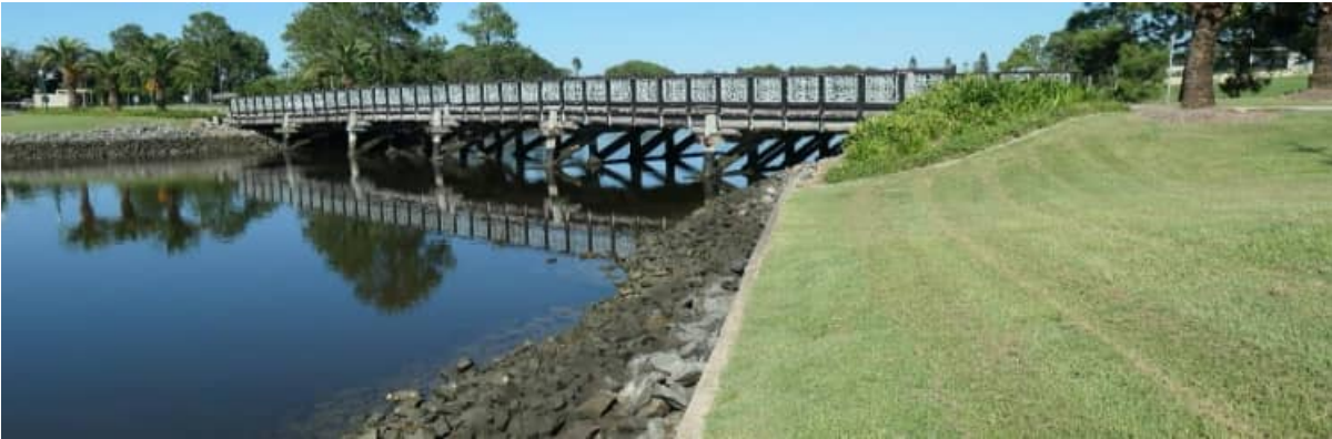
SCB-03: part view of easement / revetment wall arrangement and Western-most RCP headwall
