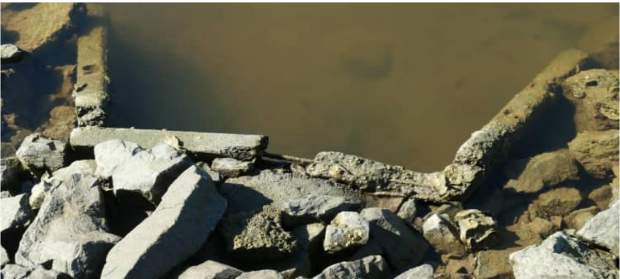
SCB-16: example view of Western-most precast headwall damage - #2
