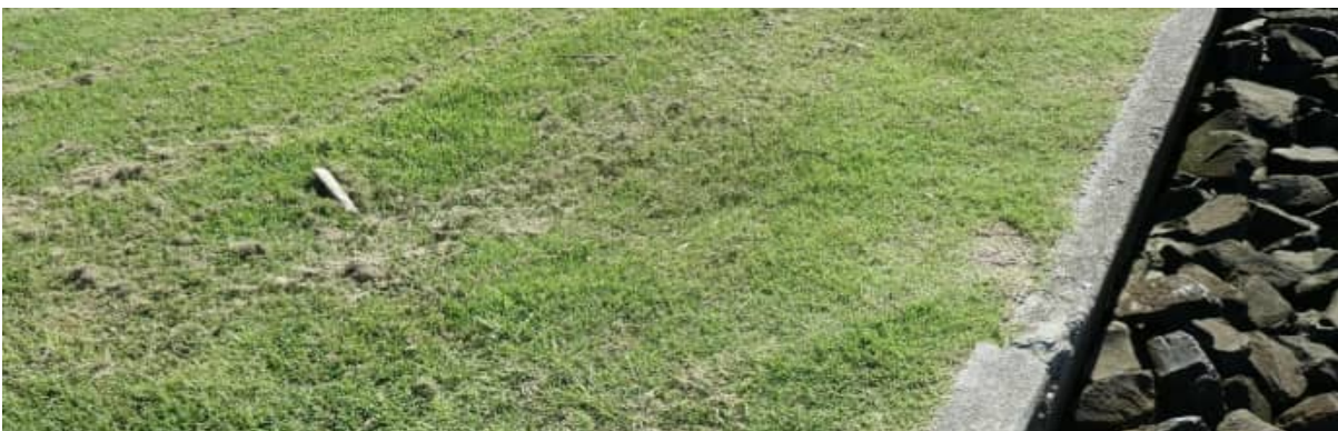
SCB-13: (relatively) nominal surface depression along the Western-most RCP alignment
