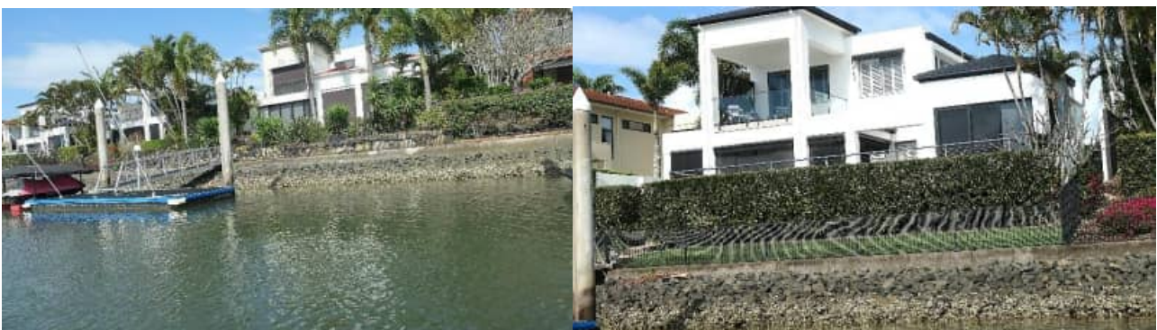
SR-59: example views of typical revetment wall / rock condition (good) to the Coomera River / 'Acacia' precinct - #3
