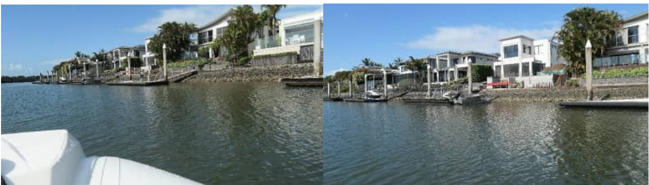
SR-58: example views of typical revetment wall / rock condition (good) to the Coomera River / 'Acacia' precinct - #2
