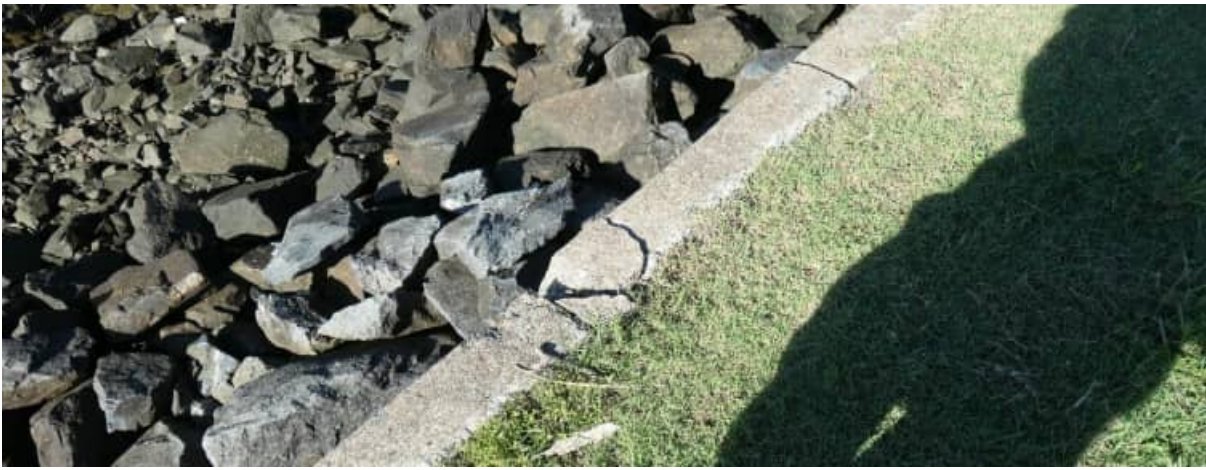
SCB-10: revetment wall construction joint (dowel) damage
