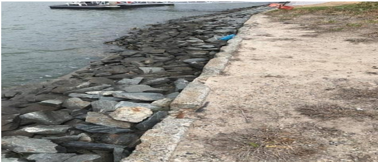
SCE-11: stem deterioration to revetment wall arrangement at easement (supplied photo) - #3
