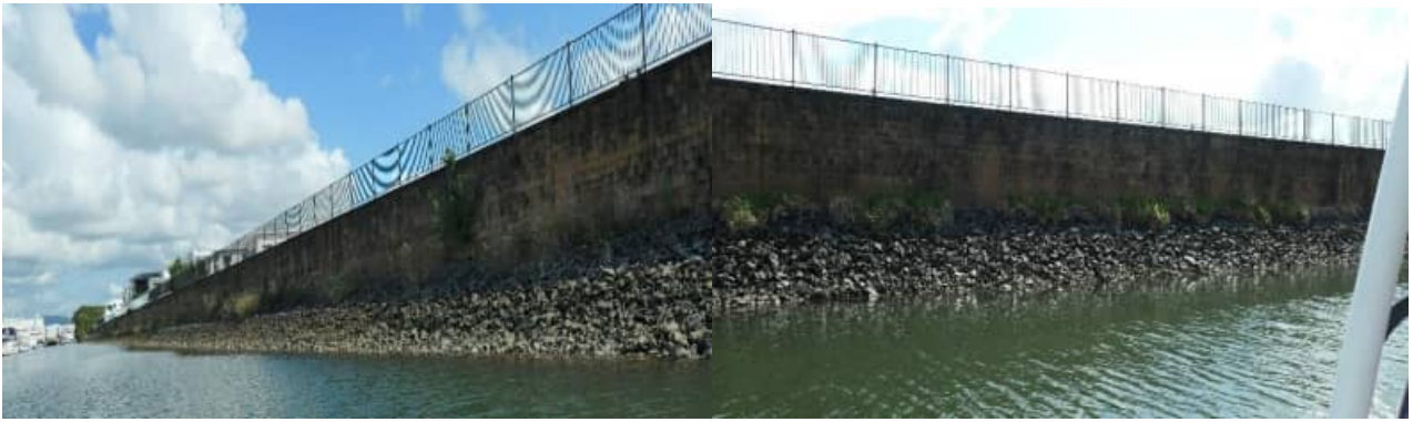
SR-76: retaining wall arrangement / rock armouring to the Southern aspect of The Point Cct
