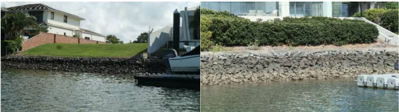
SR-69: example views of typical revetment wall / rock condition to the 'Tristania' precinct - #2
