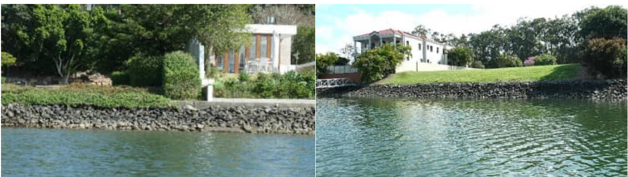
SR-69: example views of typical revetment wall / rock condition to the 'Tristania' precinct - #3
