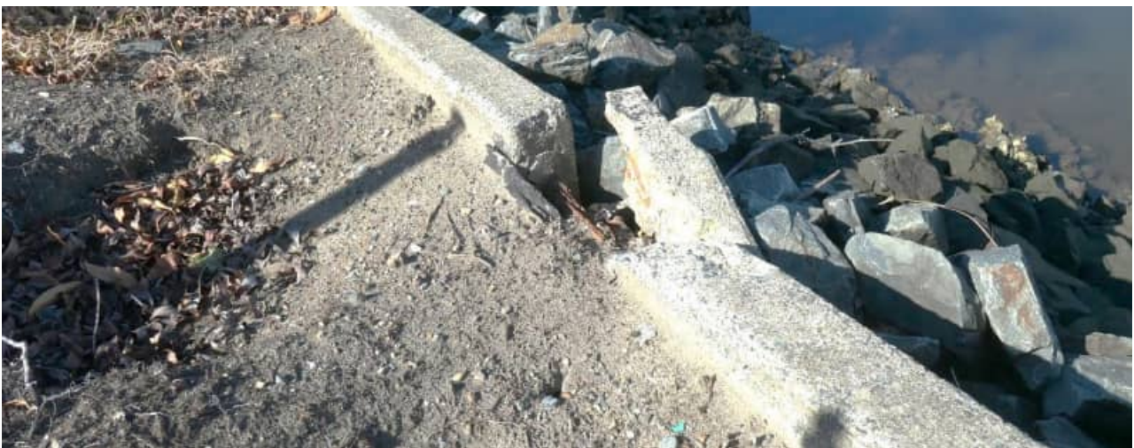
SCC-10: example view of spalling damage to the revetment wall arrangement stem - #2
