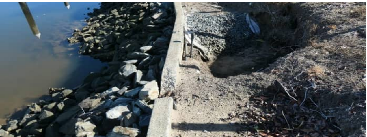
SCC-08: advanced ground subsidence issues about the stormwater RCP - #2
