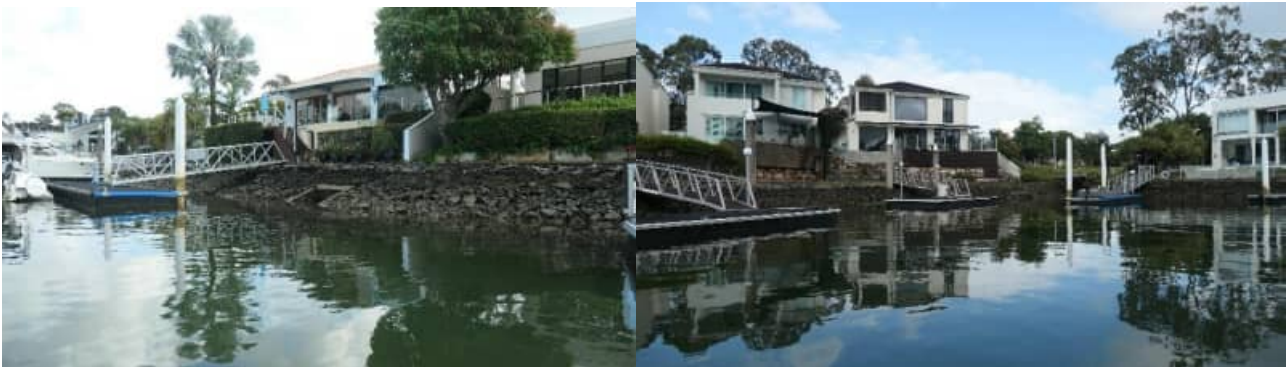
SR-48: example view of revetment wall arrangement / rock armouring to HBR3 – good condition - #2
