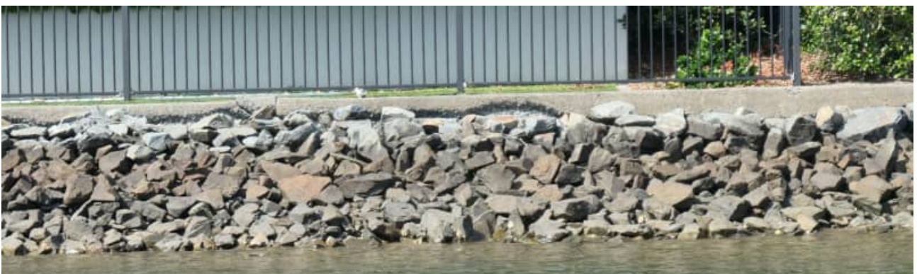
SR-67: example of advancing surface fretting / paste layer deterioration of the revetment wall arrangement stem - #3
