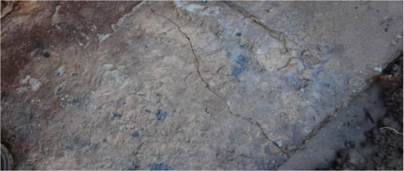
SCB-15: example view of damaged stormwater RCP replacement works (Rabaul Ave Runaway Bay) - #2
