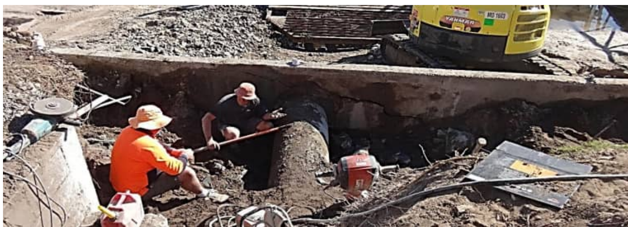
SCC-12: example view of typical subsurface stormwater RCP damage (Rabaul Ave, Runaway Bay) - #2
