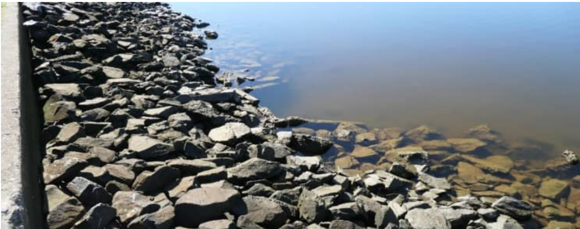
SCB-11: significantly reduced gabion rock armouring profile at Western-most outlet
