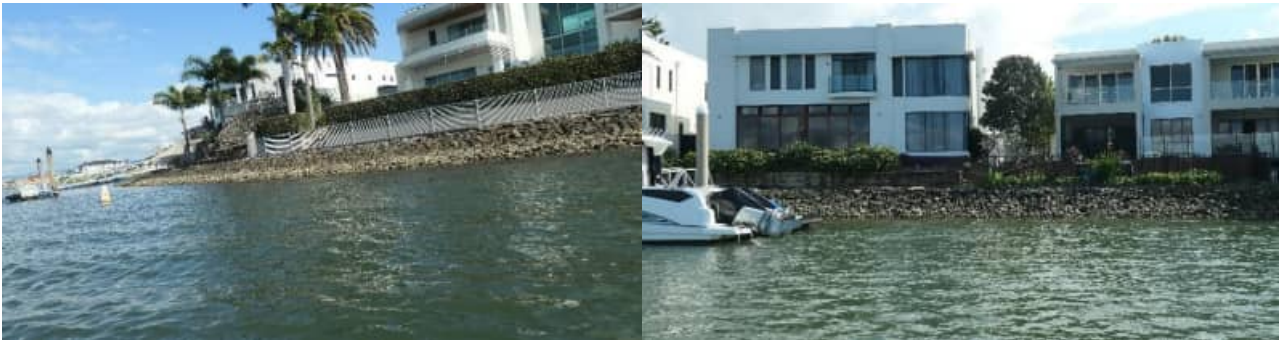
SR-68: example views of typical revetment wall / rock condition to the 'Tristania' precinct - #1
