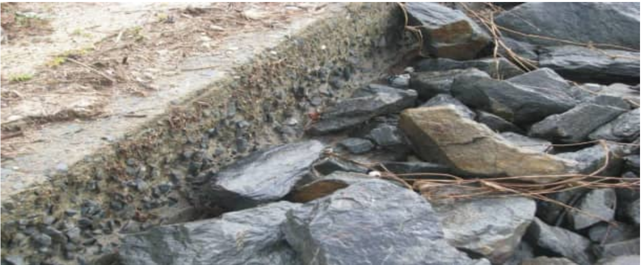
SCE-07: example of revetment wall arrangement surface deterioration of the Harbour 4 revetment wall - 2010
