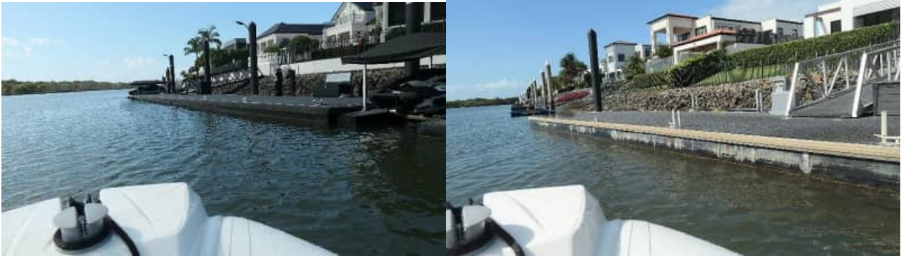
SR-57: example views of typical revetment wall / rock condition (good) to the Coomera River / 'Acacia' precinct - #1
