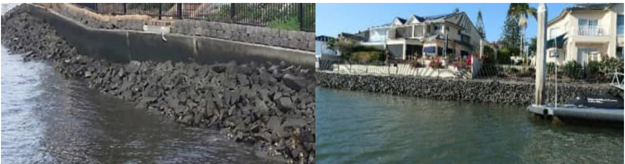
SR-05: 5318 Marine Dve North – RHS = failed wall section 2019 / LHS = replaced wall section 2024
