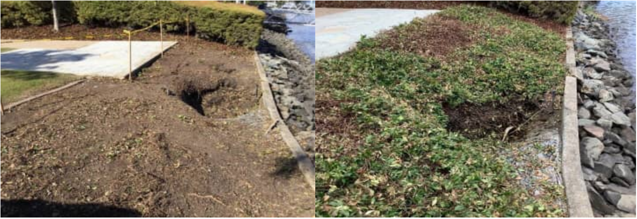
SCC-06: views of easement ground subsidence in the vicinity of the stormwater RCP (supplied photos)
