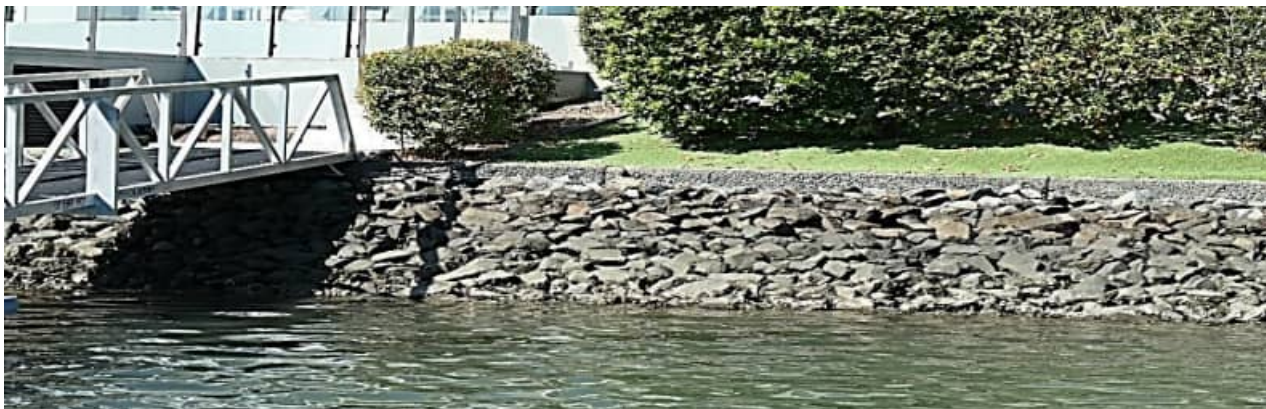
SR-60: example of typical revetment wall / rock condition (nominal surface fretting) Schotia inlet
