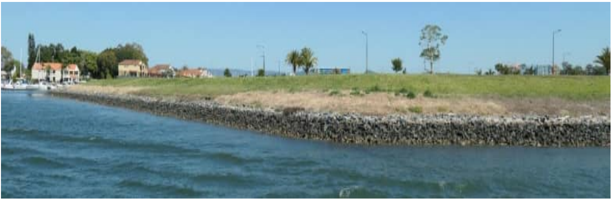
SR-77: revetment wall arrangement / rock armouring to the Eastern aspect of The Point Cct
