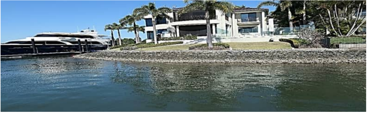
SR-63: surface fretting to revetment wall arrangement stem at 2134 The Circle - #1
