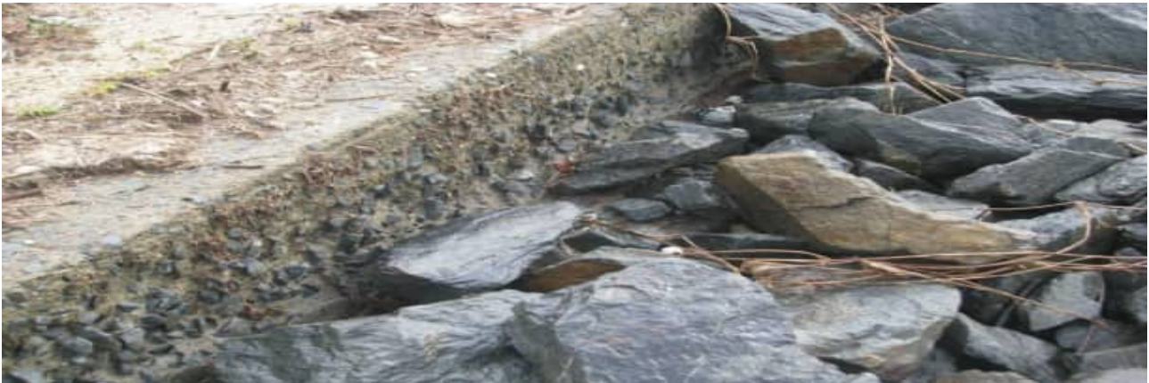
SR-65: example of revetment wall surface (paste layer) deterioration – Harbour 4 (file photo, 2011)
