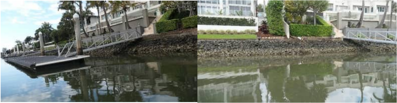
SR-27: example views of Coomera River ('Bauhinia') revetment wall and rock armouring (good) condition – #1
