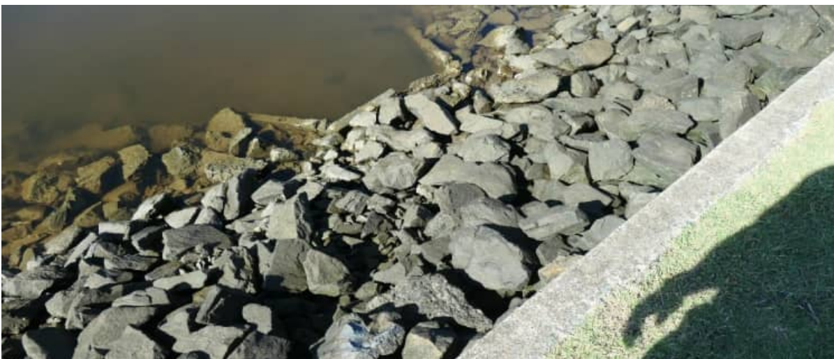
SCB-12: example view of Western-most precast headwall damage - #1
