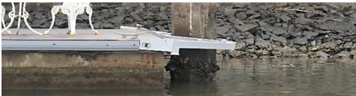
SR-09: compromised pontoon arrangement at (circa) 5302 Marine Dve Nth
